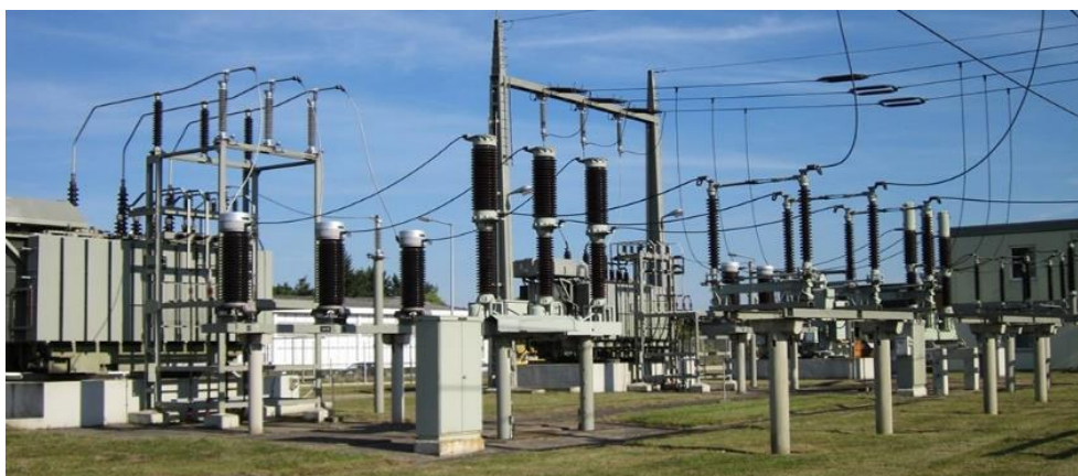
Figure 2: The High Voltage Substation
